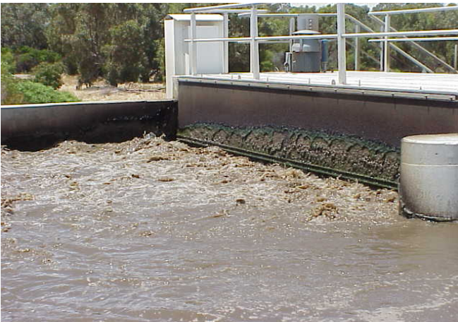
Halls Head activated sludge in oxidation ditch.
